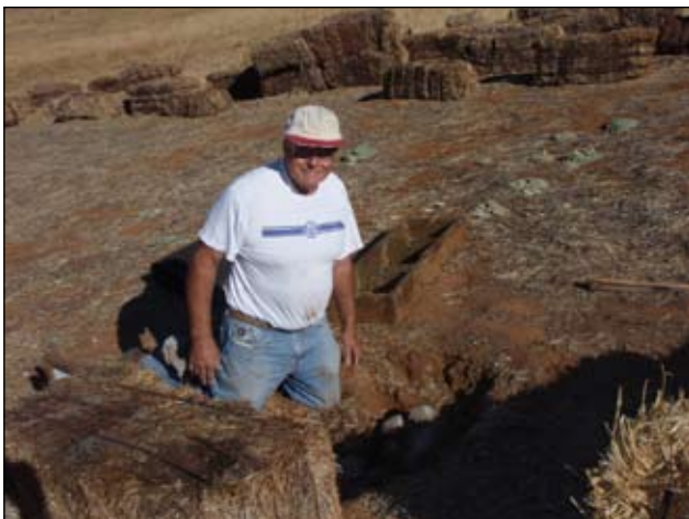
▲ Tom Grube gets the foundation ready for a sight in range target base.
